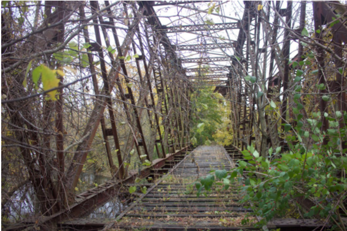
View of Caledonia's northernmost (Erie) railway bridge, facing Northwest. October 2022. This bridge has been out of commission for several years, & is currently owned by CSX.
